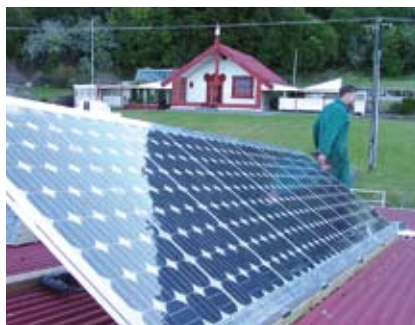
Retrofitting a house at Waipoua and installing a photovoltaic system on the roof of the Waihi wharekai. In the background, behind the whareniui, is a solar hot water system.
