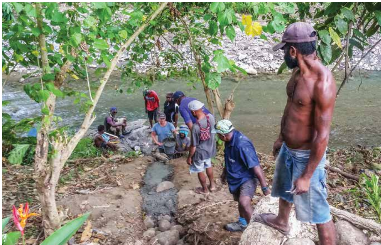
Environmental Monitoring Technician Alec Dempster and villagers install a water level gauge alongside Yalu River on the outskirts of Lae City. (Jeremy Rutherford)
