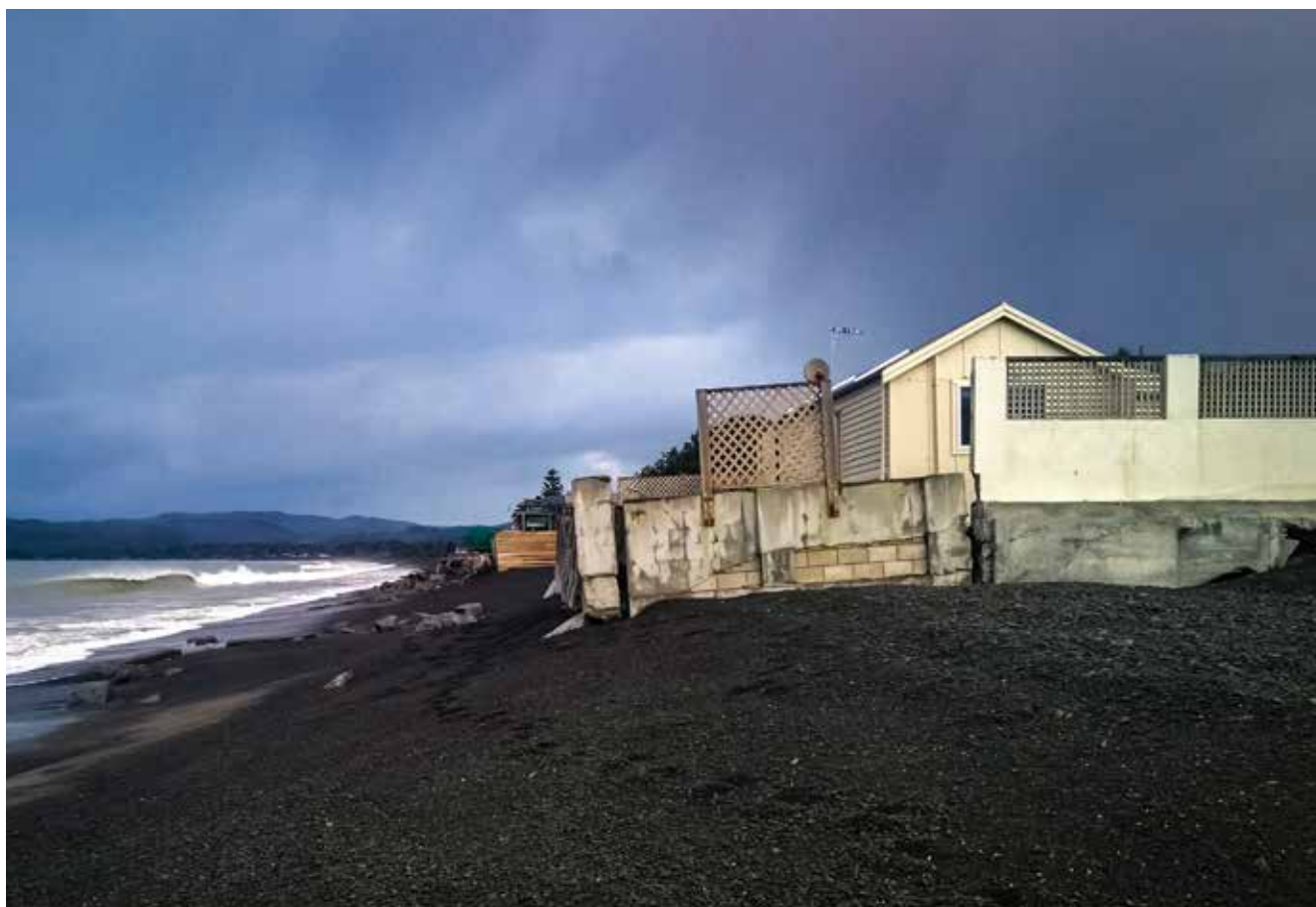
Haumoana, a coastal town just south of the Tukituki River in Hawke's Bay, is prone to coastal erosion. The shoreline is retreating at a rate between 0.3 and 0.7 metres per year. (Paula Blackett)
