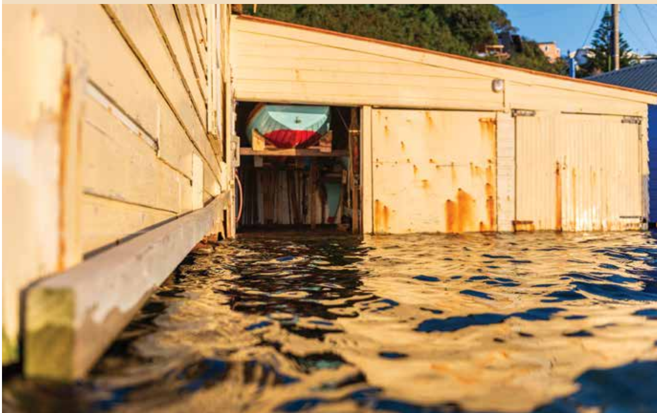
Built before sea-level rise was common knowledge – the Britannia Sea Scout' hall in Wellington's Evans Bay frequently floods during king tides and storms. (Hamish McCormick)
