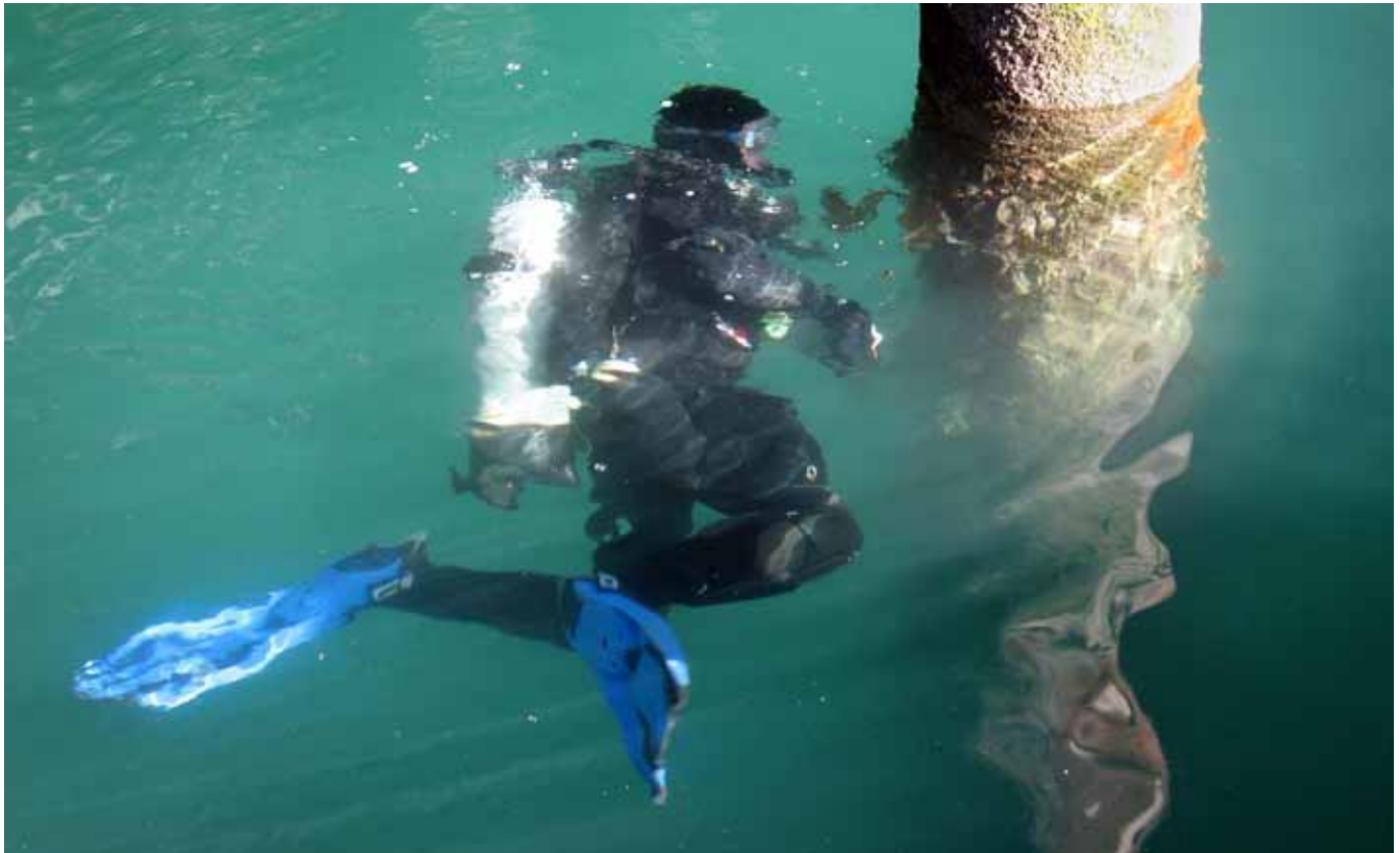
NIWA biosecurity technician Lisa Peacock checks wharf piles at Port of Lyttelton for the Mediterranean fan worm, Sabella spallanzanii , during a 2008 survey. (NIWA)
