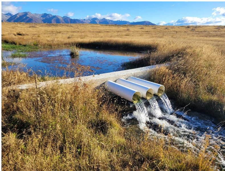
Figure 6-5: Low-head exclusion barrier installed in an unnamed spring, Waterwheel Wetland, Canterbury. The objective was to prevent trout and kōaro accessing a key bignose galaxias stronghold in the MacKenzie Basin, Canterbury. Key features of the barrier were the height (0.31 m fall from end of pipe to concrete splash pad) and downstream shallow zone (1.95 m of concrete splash pad below the pipes) to prevent trout access and the 0.62 m height and dry concrete face of the wall above the concrete pad to prevent kōaro and trout passage. Photo credit: Sjaan Bowie.
