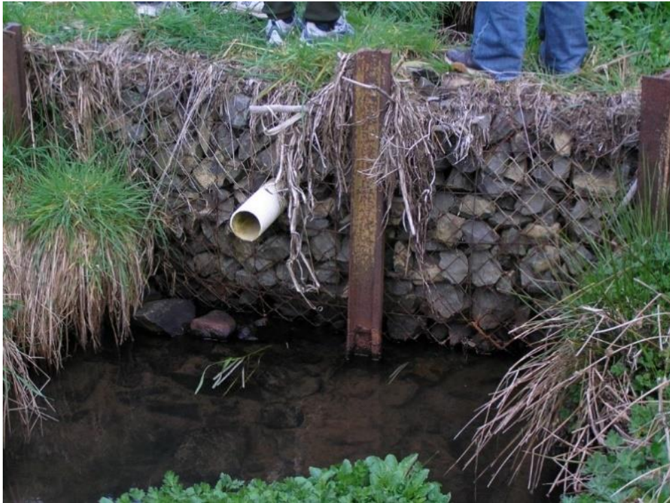
Figure 6-16: An unsuccessful gabion basket weir installed to allow migratory native fish access, while preventing trout access in Orokonui Creek, Otago. Photo credit: Sjaan Bowie.
