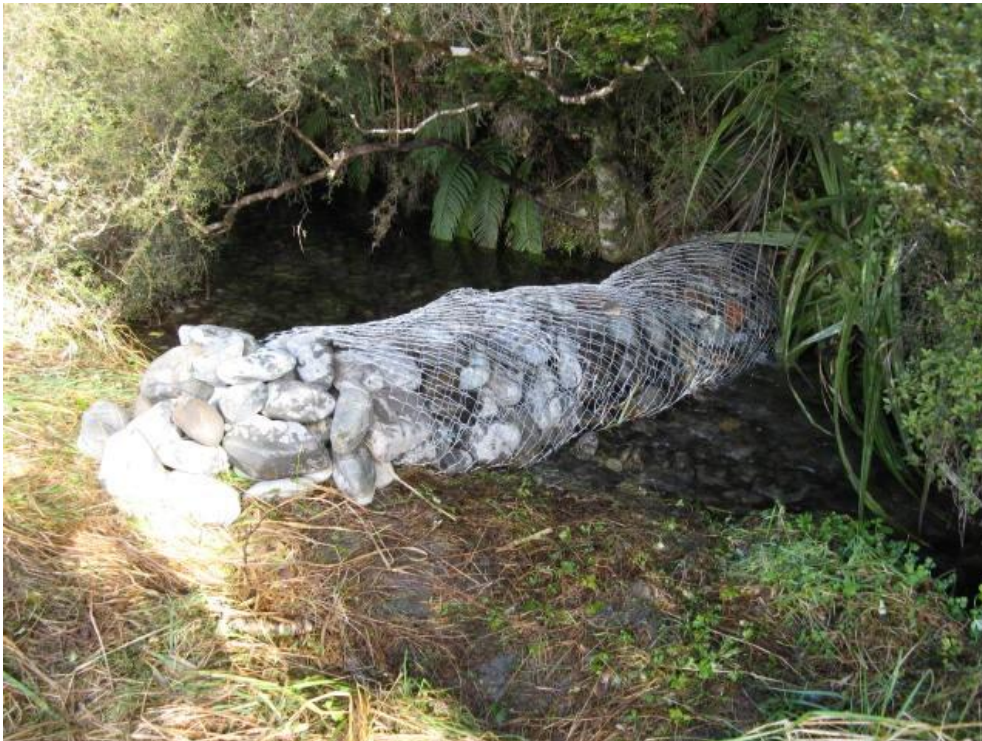
Figure 6-17: An unsuccessful gabion basket weir installed to protect a dwarf galaxias stronghold from trout in an unnamed tributary of the Maruia River, West Coast. Photo credit: Sjaan Bowie.
