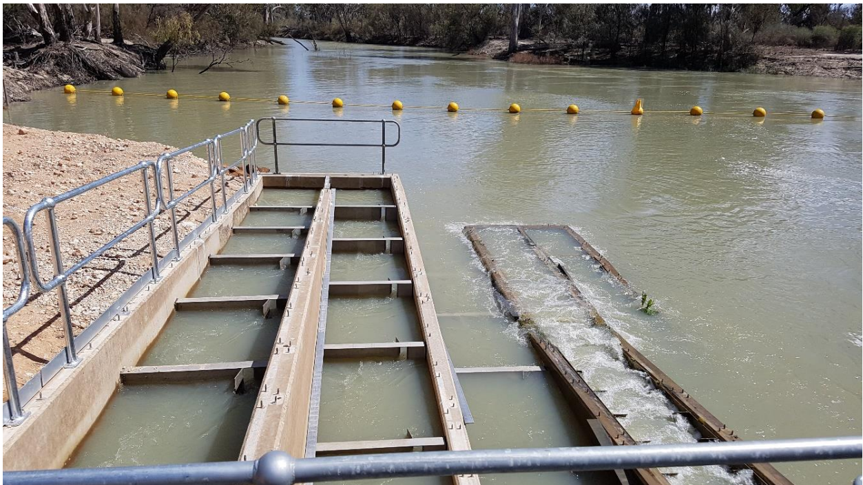
Figure 7-24: A dual Vertical Slot and Denil fishway design on Pipeclay Creek, Australia. Photo credit: Tim Marsden.
