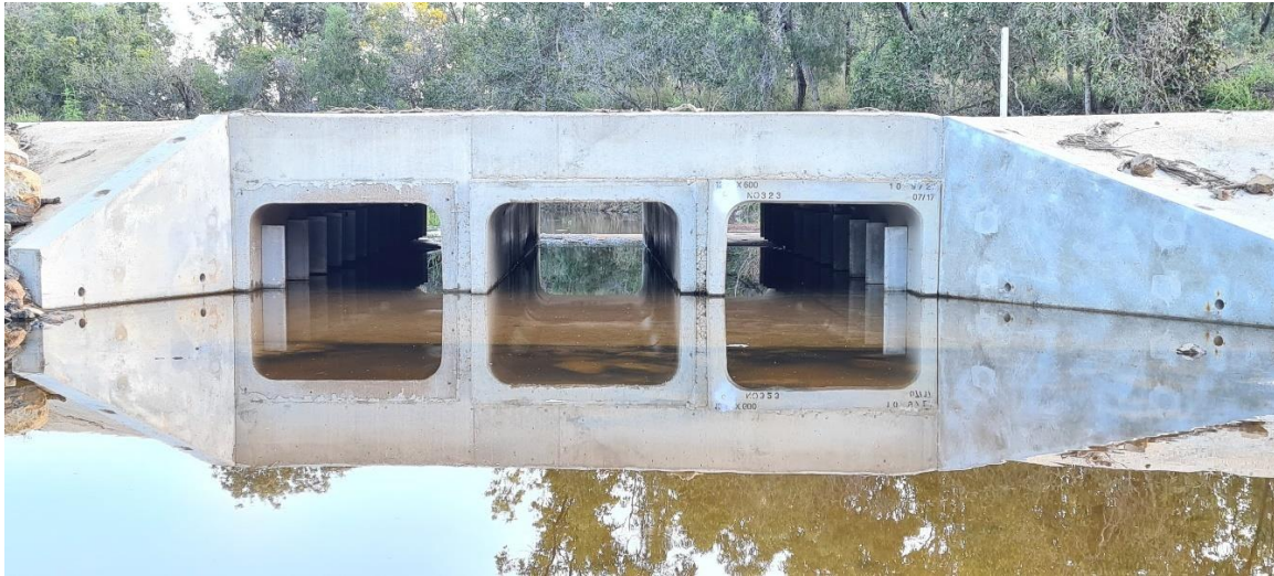
Figure 5-30: Example of vertical baffle installation on the outer walls of multi-barrel culverts. Photo credit: Tim Marsden, Australasian Fish Passage Services.
