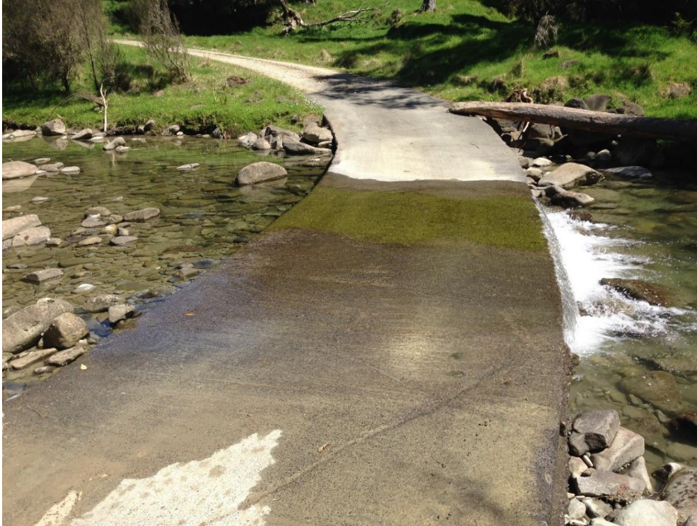
Figure 4-21: Raised roadway ford crossing. The vertical drop on the downstream side will block fish movements. Shallow water depth and elevated water velocities across the ford pavement can also impede movements.
