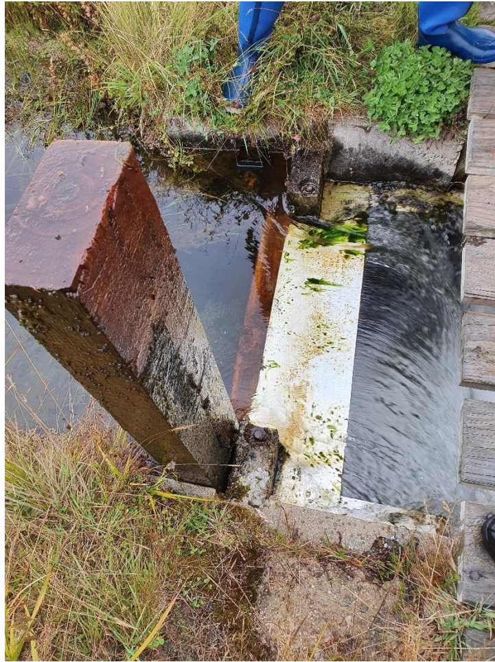
Figure 6-18: Wooden slots on the Fraser Spring exclusion barrier that can be manually removed to flush sediment and lower water levels (photo showing one removed). Photo credit: Sjaan Bowie.
