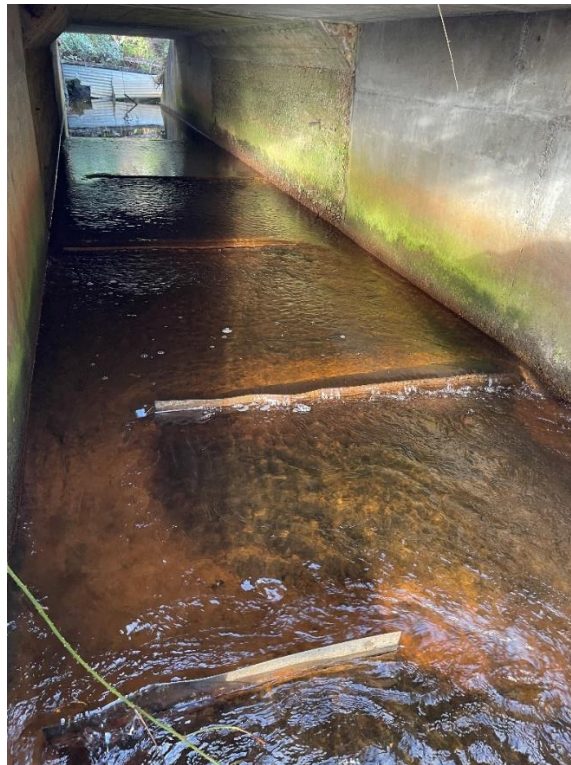
Figure J-7: Example of alternating baffles. Photo credit: Cindy Baker.
