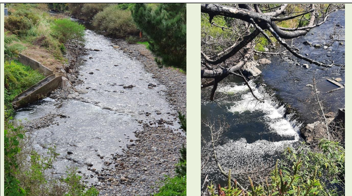
Figure 5-5: The site immediately following weir removal (Left) and two years later showing the 1 m high barrier caused by leaving the weir footings in place (Right). Photo credits: Te Korowai o Ngāruahine (left), Finnley Binsbergen (right).
