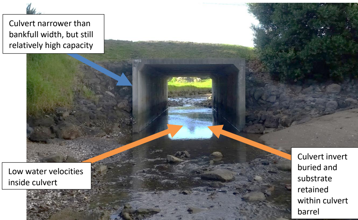
Figure B-22: Example of a culvert in a tidally influenced area. The culvert invert is embedded meaning that natural substrate is retained through the culvert. Culvert width relative to the stream bankfull width is lower than recommended, but because the culvert is in a tidal area, low water velocities will exist through the culvert during slack tide conditions. Photo credit: Bryn Quilter.
