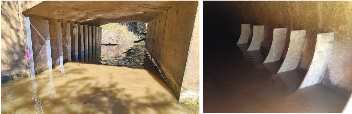
Figure 5-28: Examples of vertical baffles installed in a box culvert (left) and pipe culvert (right). Photo credit: Tim Marsden, Australasian Fish Passage Services.
