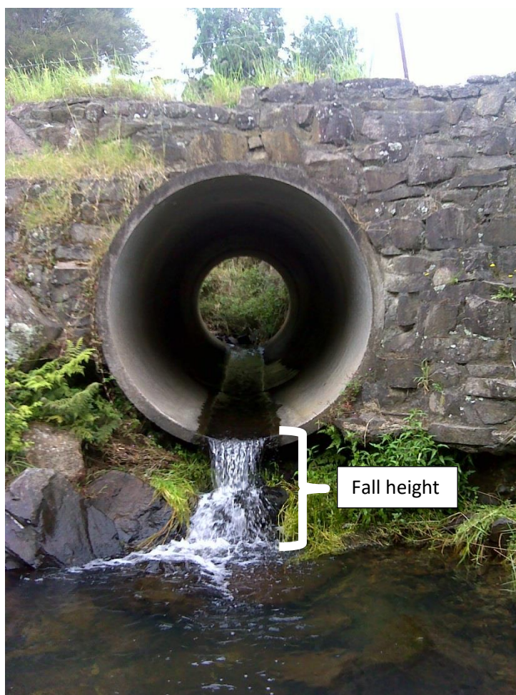
Figure B-1: Example of a perched culvert illustrating fall height.
