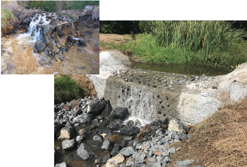
Figure 6-15: Baffled concrete weir in the lower reaches of Puketirini Stream, Waikato. A degraded weir (inset top left) was successfully preventing koi/amur carp, goldfish, perch, rudd and gambusia from accessing upstream habitats while allowing the passage of banded and giant kōkopu, and shortfin and longfin eels. To continue protecting native fish populations, the weir was remediated in 2018. Key features of the barrier include the roughness and wetted margins that desirable fish use to migrate, coupled with shallow water depths at the base of the weir to prevent large-bodied fish jumping Photo credit: Cindy Baker.
