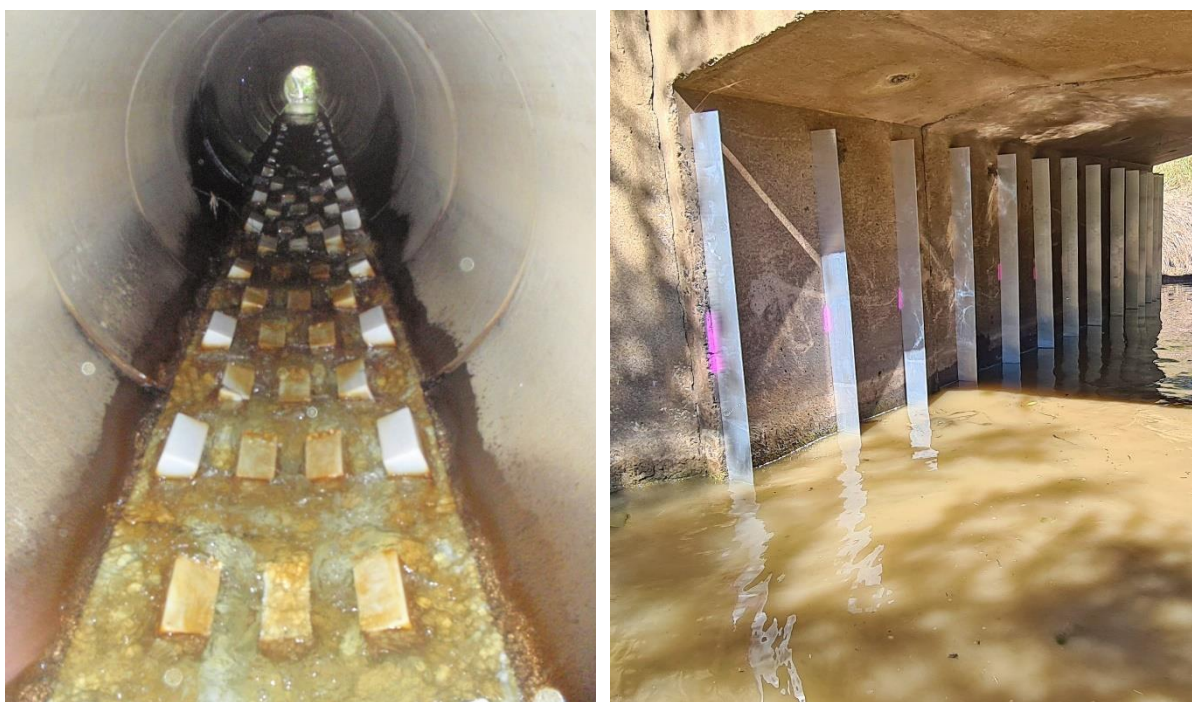
Figure 5-25: Example of spoiler baffles (left) and vertical baffles (right) installed inside culverts. Spoiler baffles credit: NIWA. Vertical baffles credit: Tim Marsden, Australasian Fish Passage Services.
