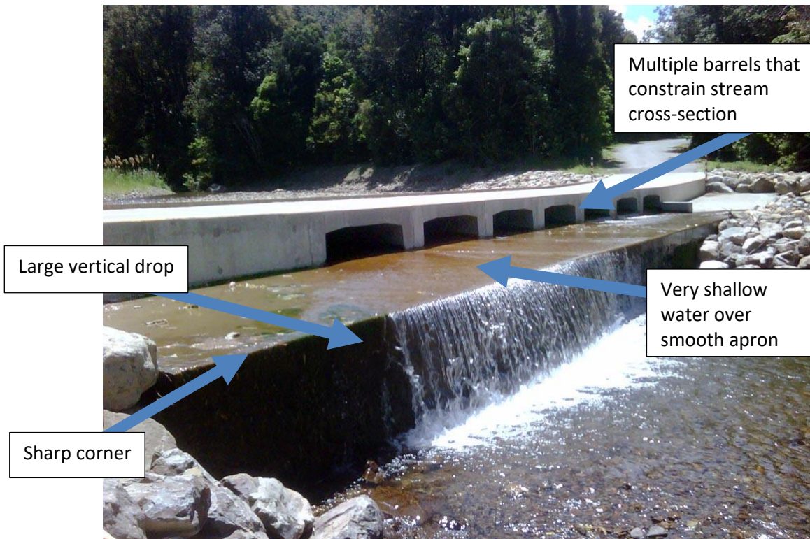
Figure B-18: An example of a drift-deck ford. This is a significant barrier to fish due to the large fall height on the downstream side of the structure. Passage may also be impeded by the sharp corner on the edge of the apron, shallow water, and high water velocities during high flow.
