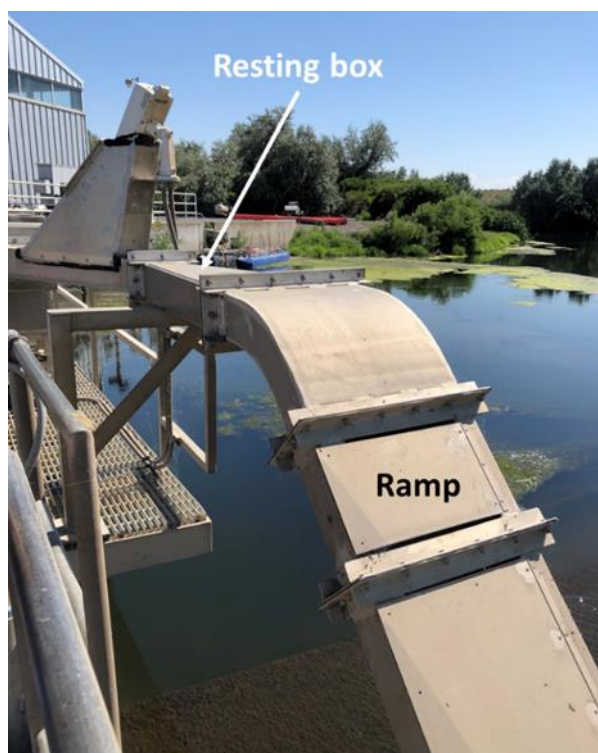
Figure 7-12: Example of a resting box in a LPS designed for Pacific lamprey passage at Three Miles Falls Dam, Umatilla River, Oregon. Photo credit: Cindy Baker.
