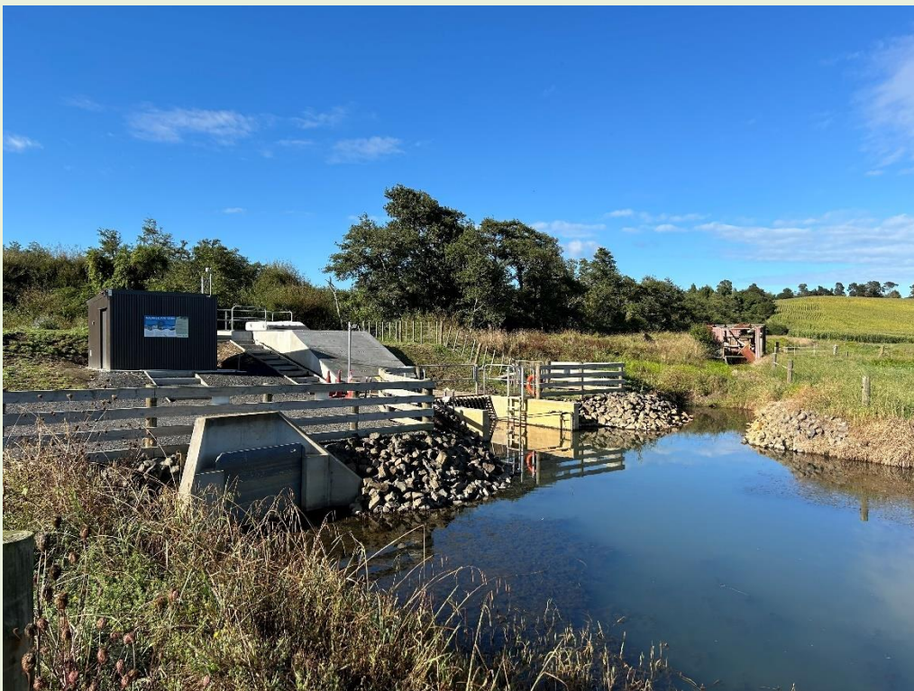
Figure 4-28: The new Mangawhero enclosed Archimedes screw pump site near Aka Aka. Photo credit: Paul Franklin.
