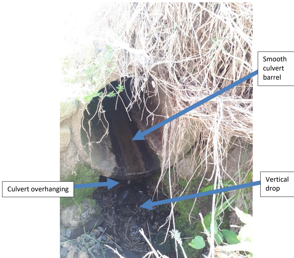
Figure B-15: Fish passage will be impeded by the fall height and undercut at the culvert outlet. The smooth culvert barrel will also lead to higher water velocities and limit fish movements under higher flows. Photo credit: Megan Brown.
