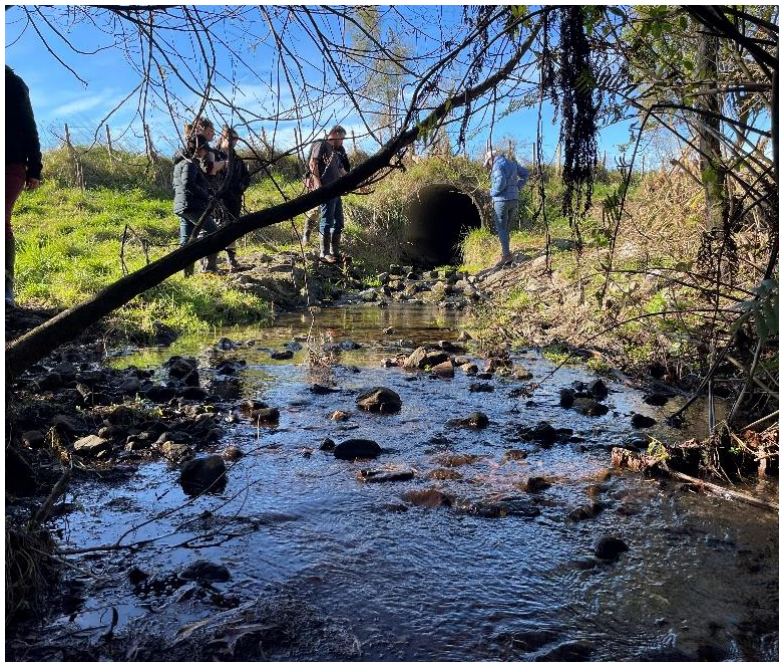
Figure 5-15: An example of a grouted concrete rock ramp below a culvert in the Manawatu-Wanganui region. Top, as built in 2014. Bottom, a decade later in 2024. Concrete is used to prevent water seepage between rocks and is shaped to provide a low flow channel and resting pools to facilitate upstream passage. Photo credit: Cindy Baker.
