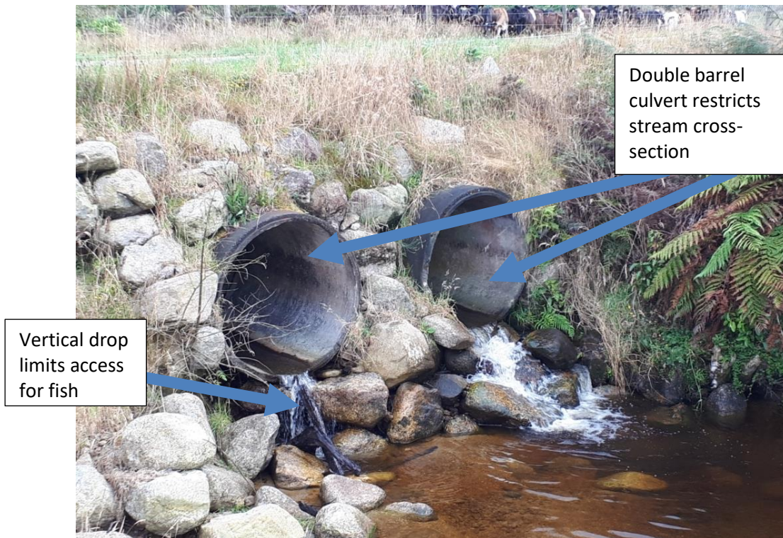
Figure B-16: A double barrel culvert where passage will be impeded by the fall height at the culvert outlet. Passage for climbing fish species may be possible over the rocks below the culvert in the right of the picture. Photo credit: Sam Ammon.
