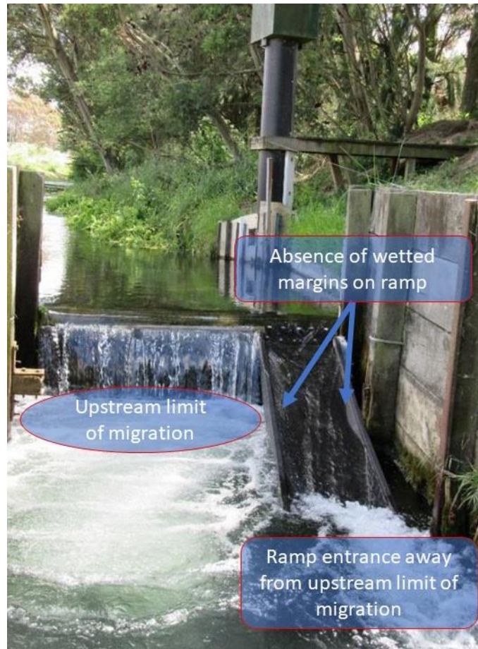
Figure 5-23: Example of a partial-width floating ramp installation. The ramp entrance is located away from the upstream limit of migration which will reduce entrance efficiency. Furthermore, under the pictured flows there is too much flow going down the ramp meaning there are no wetted margins maintained. Photo modified from Fake (2018).
