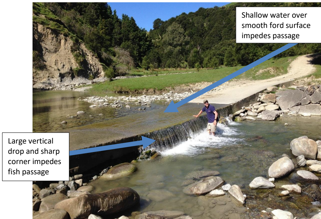
Figure B-21: The fall height on this ford on the Te Arai River is a significant impediment to the upstream passage of fish. Photo credit: Paul Franklin.
