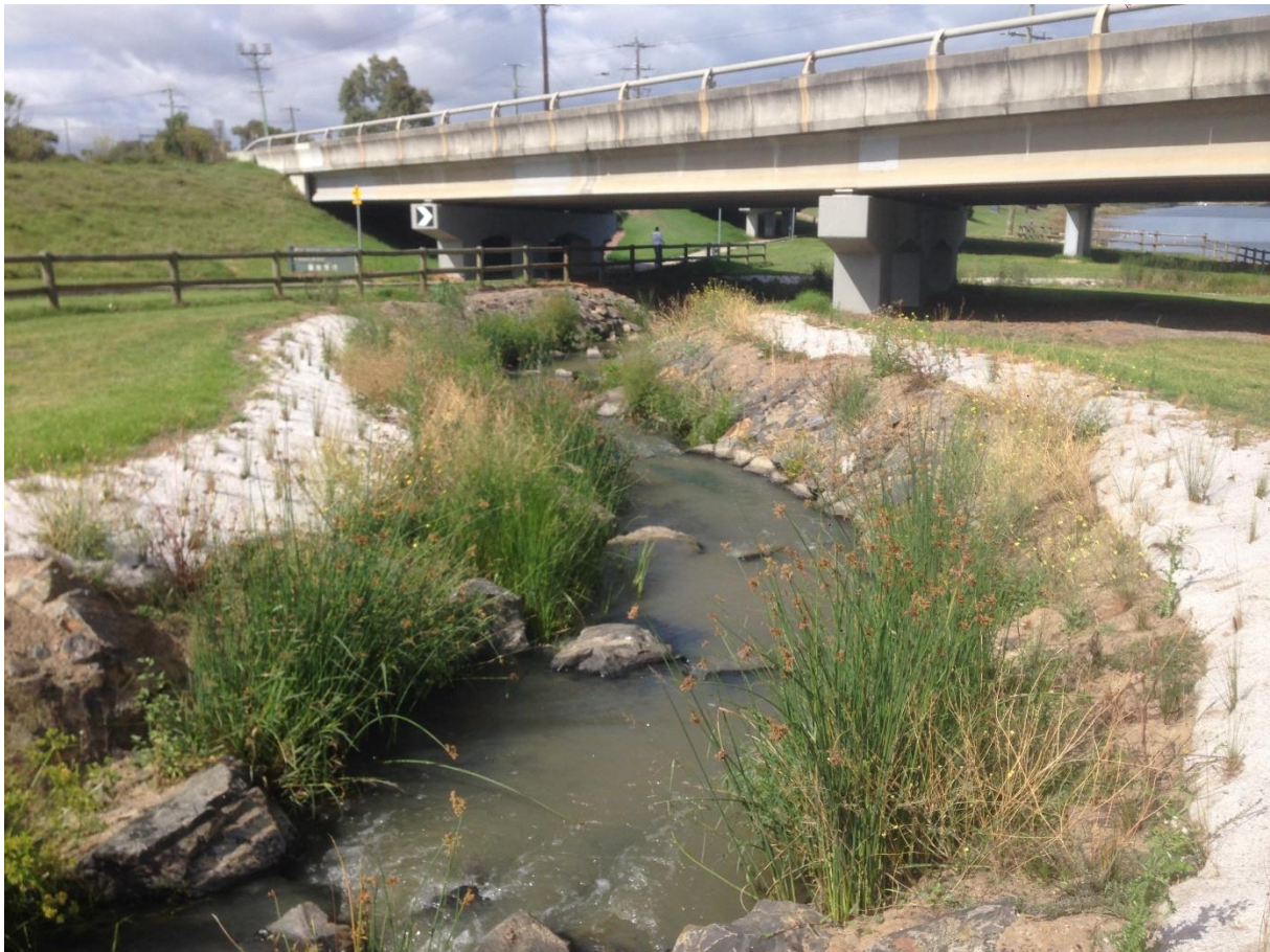
Figure 5-1: Example of a low gradient nature-like rock ramp fishway on the Patterson River near Melbourne, Australia. Photo: Paul Franklin.
