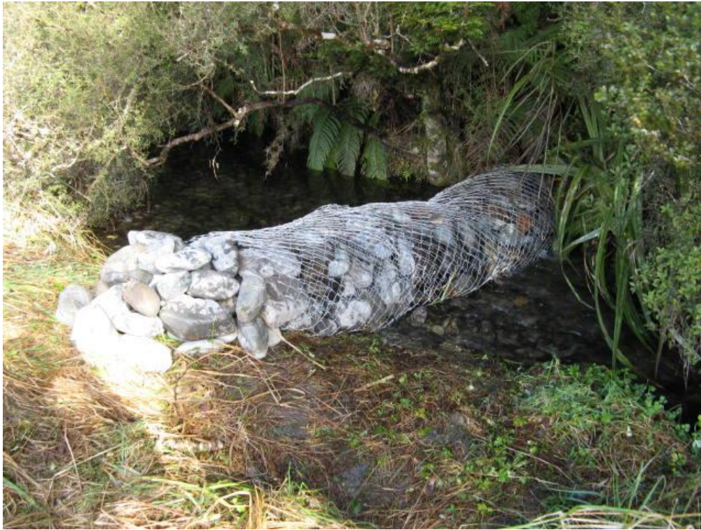
Figure 6-12: An unsuccessful gabion basket weir installed to protect a dwarf galaxias stronghold from trout in an unnamed tributary of the Maruia River, West Coast. Credit: Sjaan Bowie.
