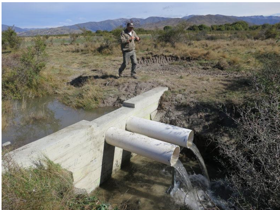
Figure 6-4: Built barrier installed in an unnamed spring of the Ahuriri. The objective was to prevent trout accessing a key lowland longjaw galaxias stronghold in the MacKenzie Basin, Canterbury. Credit: Dean Nelson (DOC).
