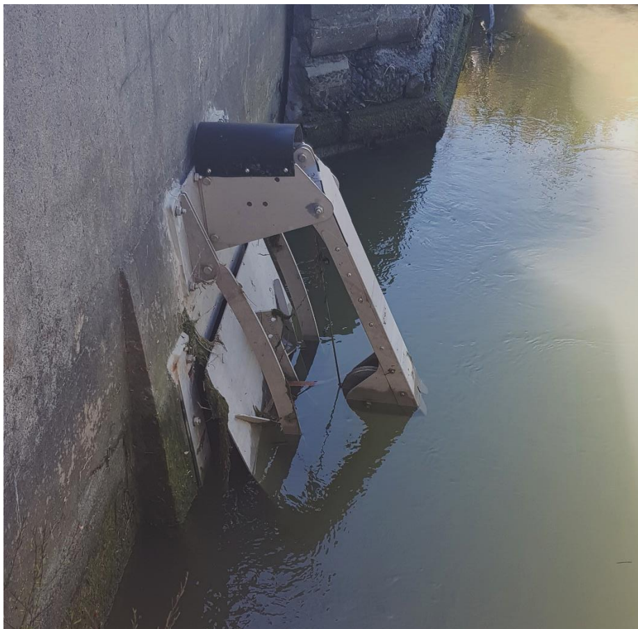
Figure 5-12: A tide gate retrofitted with a fish friendly counter weight system in Christchurch. Credit: Paul Franklin.
