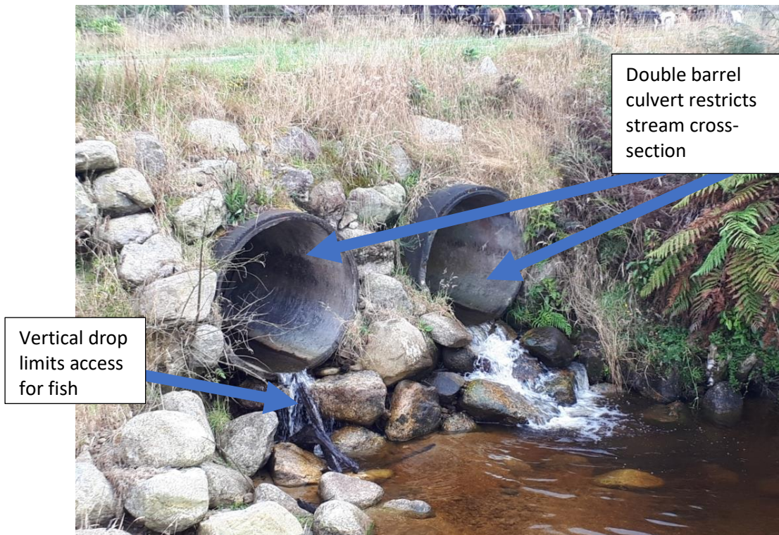
Figure E-16: A double barrel culvert where passage will be impeded by the fall height at the culvert outlet. Passage for climbing fish species may be possible over the rocks below the culvert in the right of the picture. Credit: Sam Ammon.
