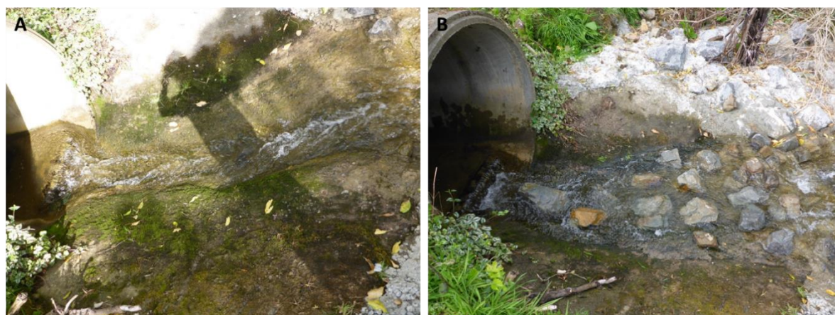
Figure I-3: Culvert apron at Upper Kingston Road. A, unmodified. B, modified using boulders as baffling elements.
