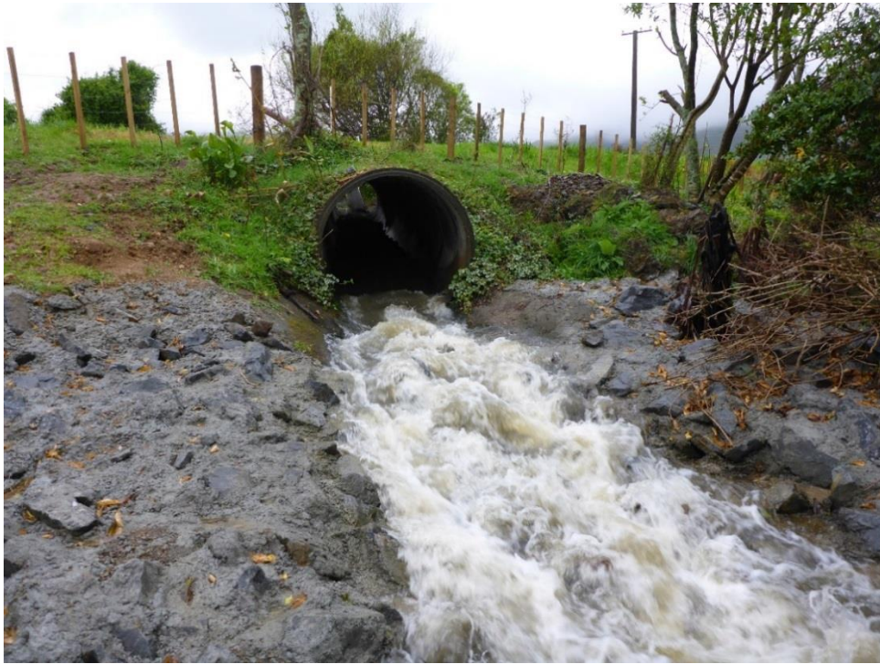
Figure I-11: Flow through the culvert and over the rock-ramp at the conclusion of Trial 3.
