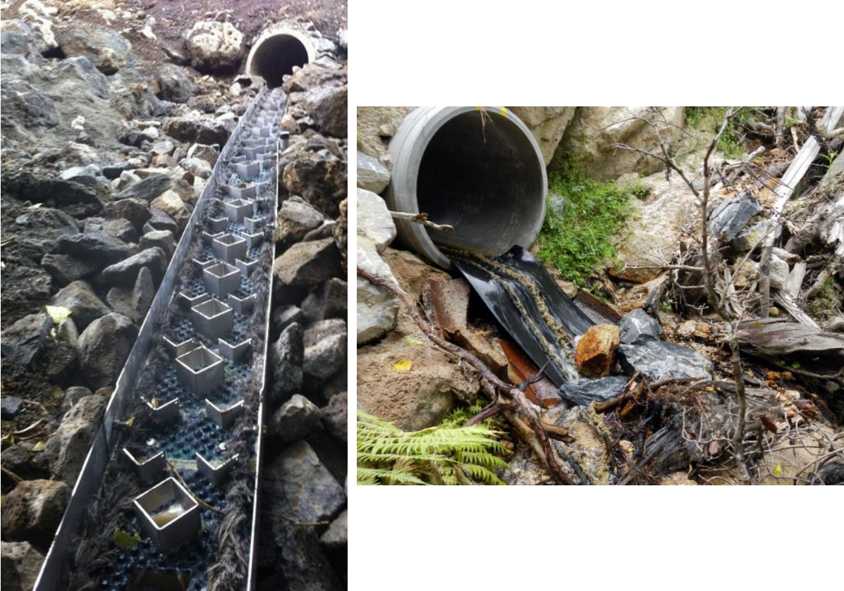
Figure 8-1: Examples of novel fish passage remediation solutions for perched culverts. Left: An example of a novel fish ladder design. Right: Conveyor belt rubber being used as a fish ramp alongside mussel spat ropes.
