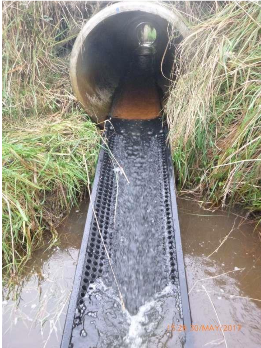
Figure 5-5: Example of an artificial fish ramp installed at a perched culvert in Southland. Note that a shallow wetted margin is maintained on both sides of the ramp. Photo: James Dare.
