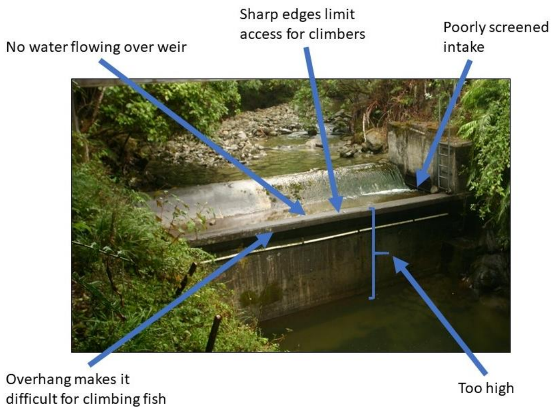
Figure 2-3: An example of an intake weir identifying features unsuitable for fish passage.
