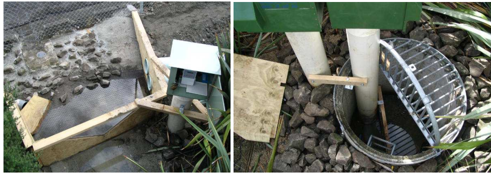
Figure 41 Monitoring instruments were installed at the raingarden inlet (left) and outlet (right) to record inflow and outflow and to sample stormwater for chemical analysis. Photo by Pete Pattinson, 2006.
