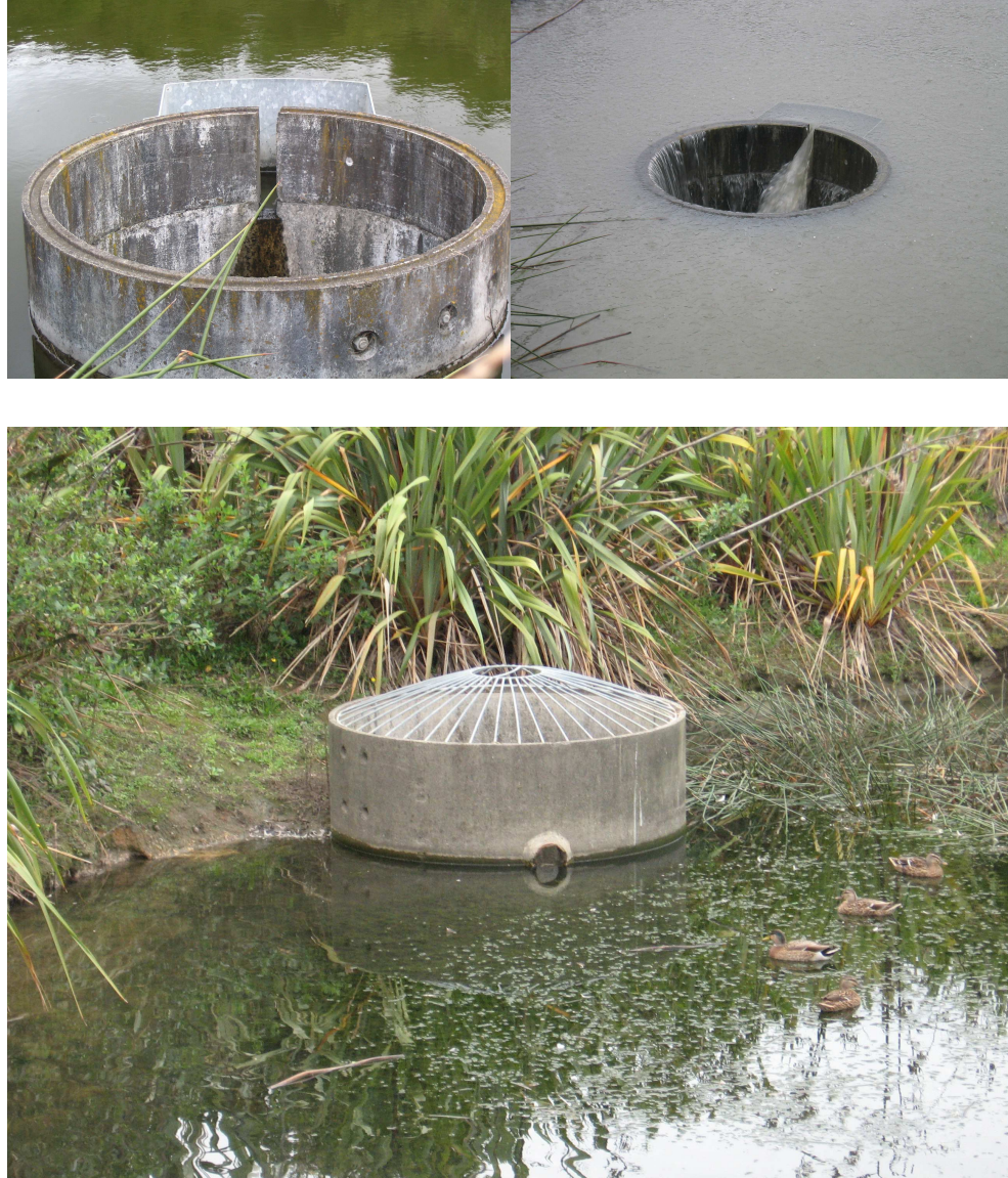
Figure 31 The outlet standpipes for the Silverdale (above, high and low flow conditions) and Te Atatu (bottom, low flow) ponds showing the secondary outlets for extended detention.
