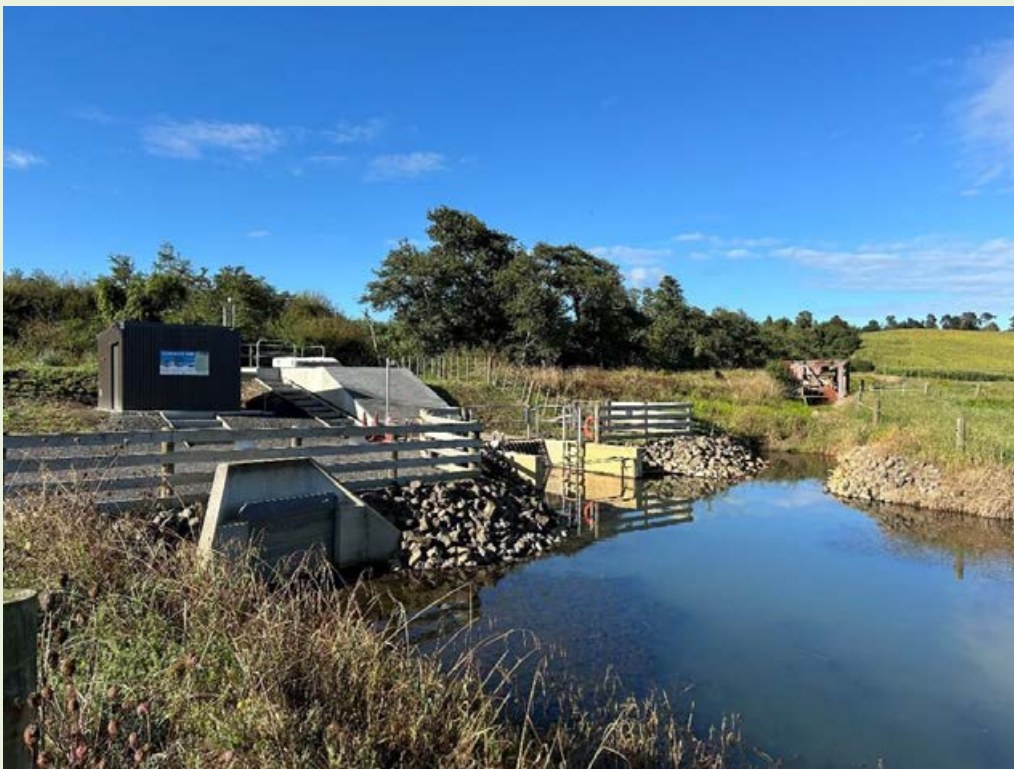
Figure 4-28: The new Mangawhero enclosed Archimedes screw pump site near Aka Aka. Photo credit: Paul Franklin.
