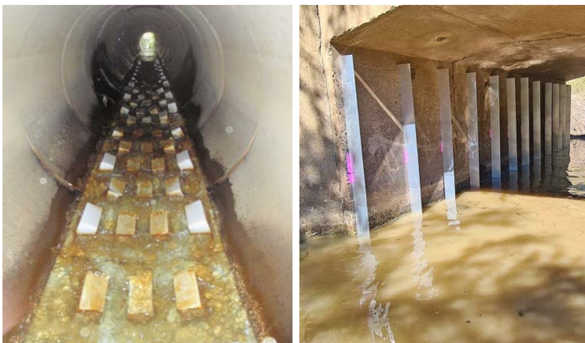
Figure 5-25: Example of spoiler baffles (left) and vertical baffles (right) installed inside culverts. Spoiler baffles credit: NIWA. Vertical baffles credit: Tim Marsden, Australasian Fish Passage Services.
