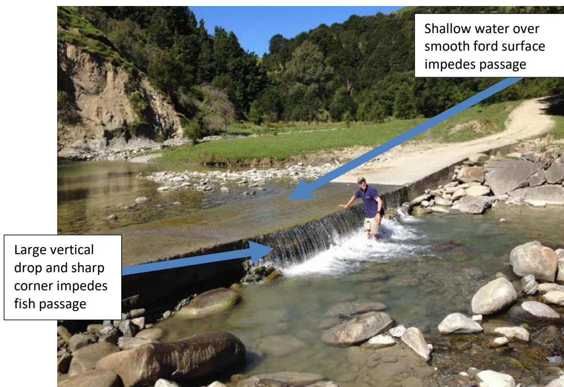
Figure B-21: The fall height on this ford on the Te Arai River is a significant impediment to the upstream passage of fish. Photo credit: Paul Franklin.
