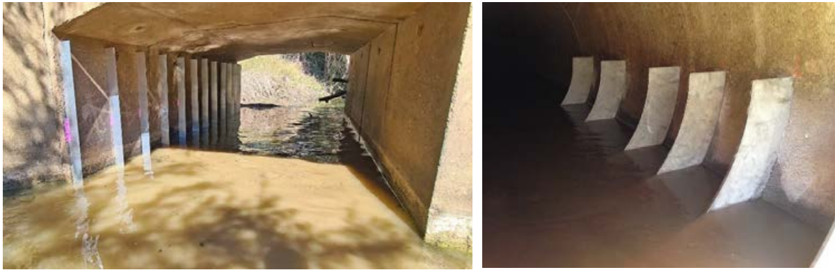
Figure 5-28: Examples of vertical baffles installed in a box culvert (left) and pipe culvert (right). Photo credit: Tim Marsden, Australasian Fish Passage Services.
