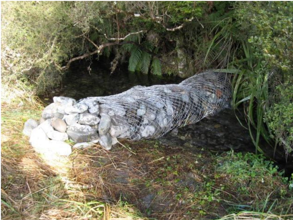
Figure 6-17: An unsuccessful gabion basket weir installed to protect a dwarf galaxias stronghold from trout in an unnamed tributary of the Maruia River, West Coast. Photo credit: Sjaan Bowie.
