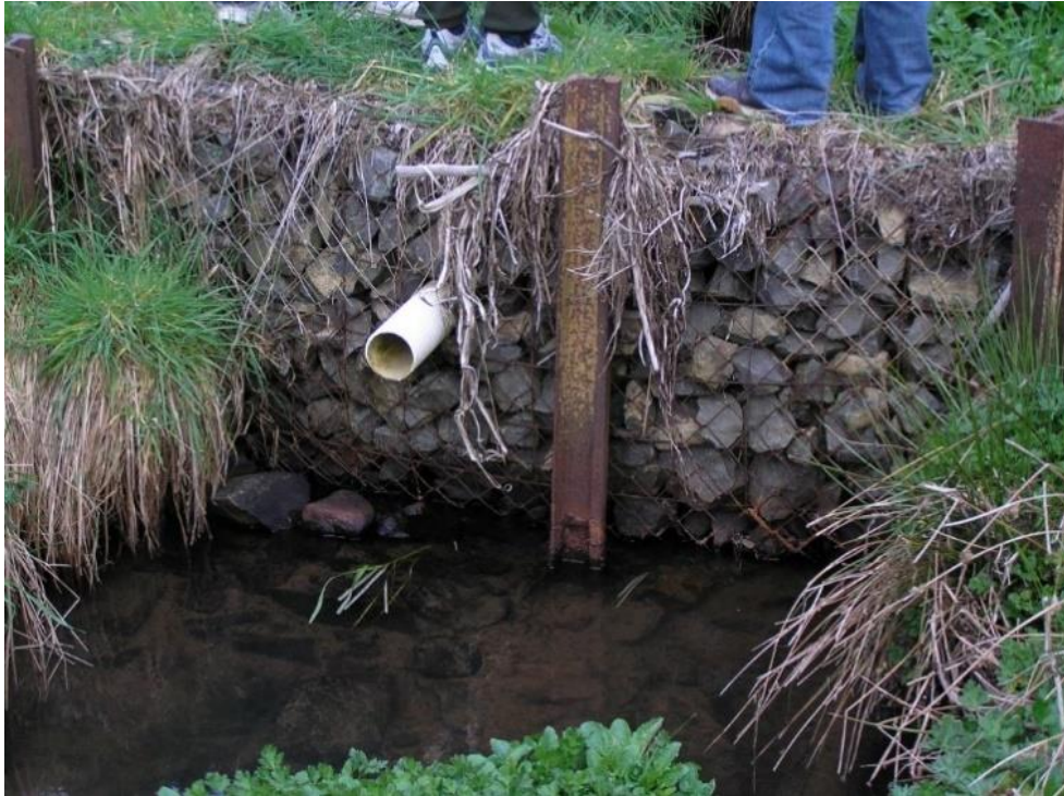
Figure 6-16: An unsuccessful gabion basket weir installed to allow migratory native fish access, while preventing trout access in Orokonui Creek, Otago. Photo credit: Sjaan Bowie.
