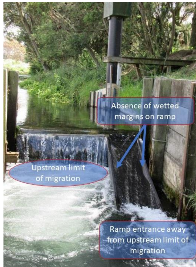
Figure 5-23: Example of a partial-width floating ramp installation. The ramp entrance is located away from the upstream limit of migration which will reduce entrance efficiency. Furthermore, under the pictured flows there is too much flow going down the ramp meaning there are no wetted margins maintained. Photo modified from Fake (2018).
