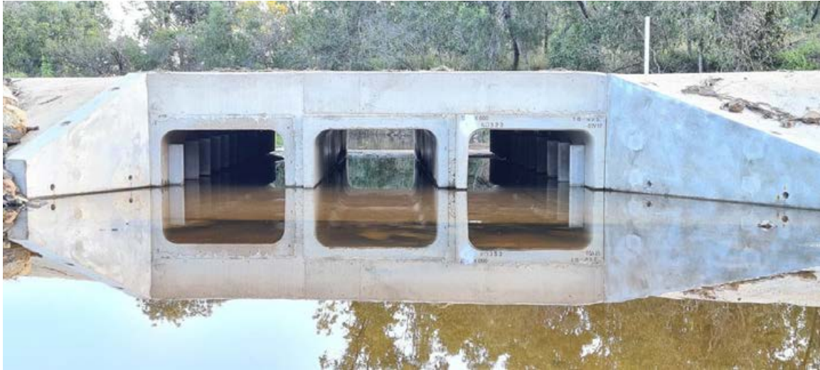
Figure 5-30: Example of vertical baffle installation on the outer walls of multi-barrel culverts. Photo credit: Tim Marsden, Australasian Fish Passage Services.
