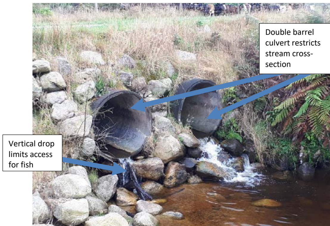
Figure B-16: A double barrel culvert where passage will be impeded by the fall height at the culvert outlet. Passage for climbing fish species may be possible over the rocks below the culvert in the right of the picture. Photo credit: Sam Ammon.
