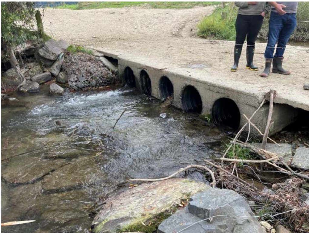
Figure 4-22: Raised roadway ford crossing with culverts. At low flows, water passes through the culverts in the ford, rather than over the roadway. The small culverts used in this ford severely constrict the river channel and will result in accelerated water velocities through the culvert barrel that may be impassable to fish.
