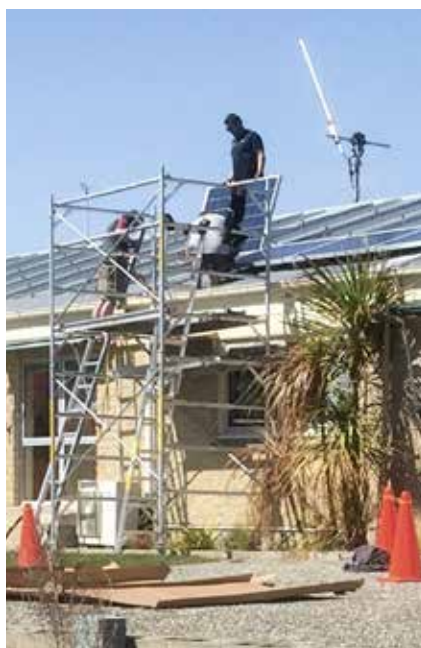
Solar panels being installed at Lauder to measure the effects of atmosphere on solar energy production. (Ben Liley)
