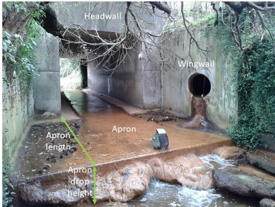
Figure E-1: Example of a culvert with an integrated headwall, wingwalls and apron.
