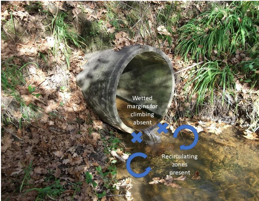
Figure C-5: Example of where low velocity recirculation zones are present, but wetted climbing margins are absent.
